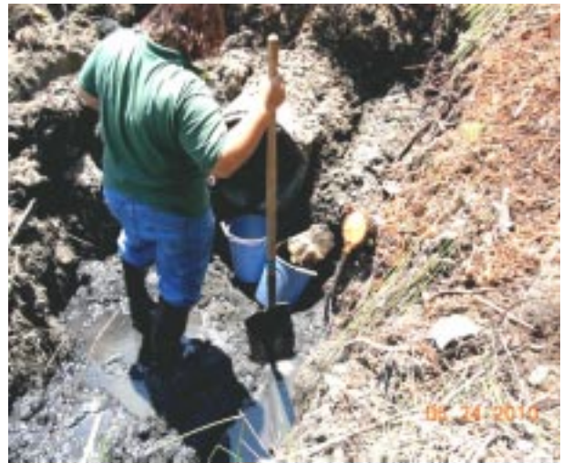
Manager Drake places buckets under two drains to catch effluent.
