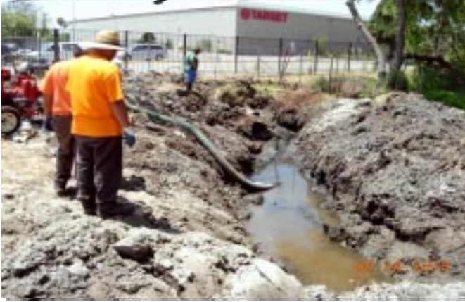
Manager Tracy Drake (in background) and two city workers pump effluent from new “drainage basin” at southwest corner of Preserve.
