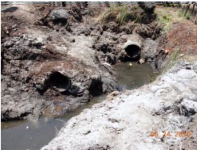
Our three incoming drains: large drain at lower left is from south, under Sepulveda; large drain at right is under Madrona from carwash; to its right is the smaller, ‘mystery’ drain.
