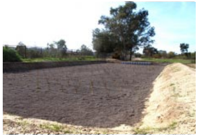
Biofilter complete with special Vetiver grass from India planted. Twelve pipes protruding at far end supply water that has been pumped up from the sump.
