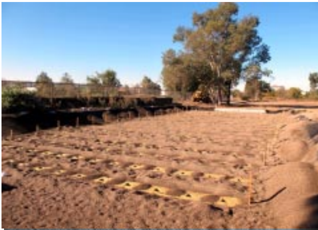
The hole is then filled with adsorbent gravel-like stone plus rows of special absorbent media (lighter boxes) in which grass will be planted.
