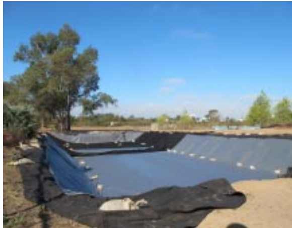
Construction of new subsurface biofilter begins with a 110'x35'x6' hole, lined with fabric to form water barrier.
